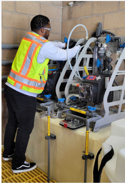
Figure 1. Performing a drawdown is one of the most reliable ways to calibrate a pump.
